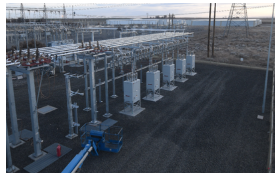
Part of the expanded Franklin Substation low side bus with additional feeders.
