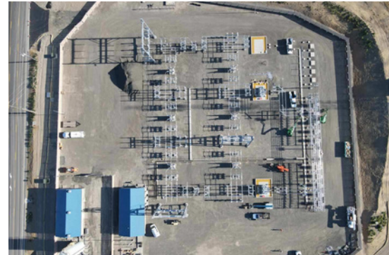
Aerial view of the Railroad Avenue substation.
