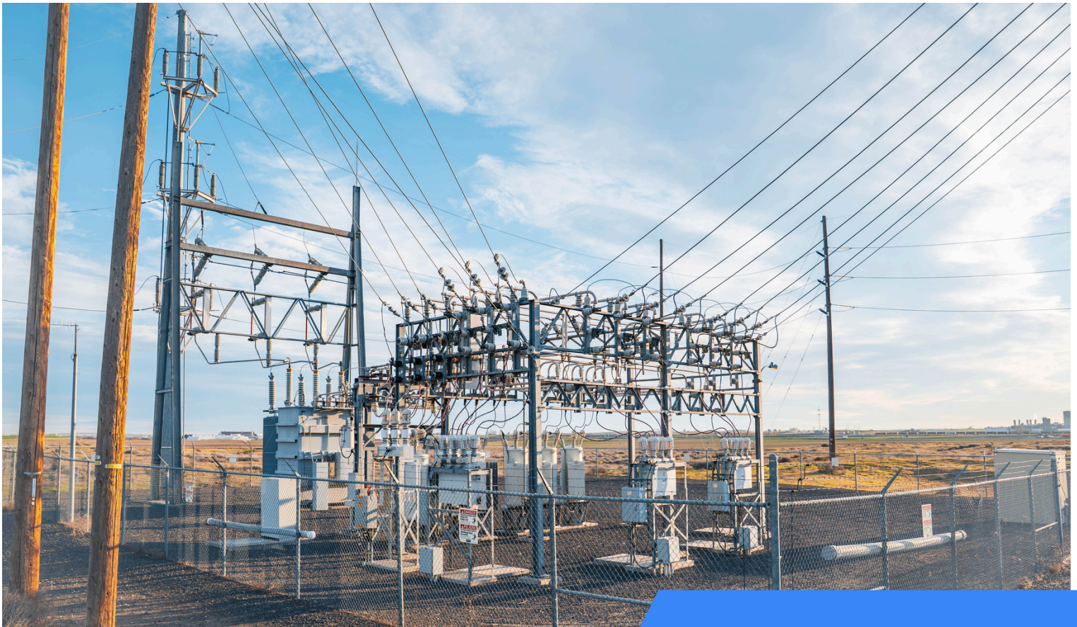
North Pasco Substation
